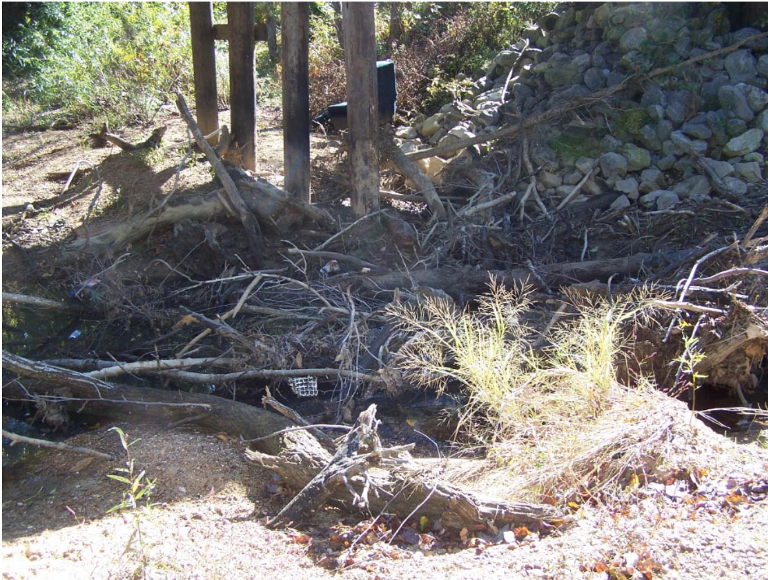
042-C252 SCOUR & DRIFT AT BENT 2 10/20/2011
