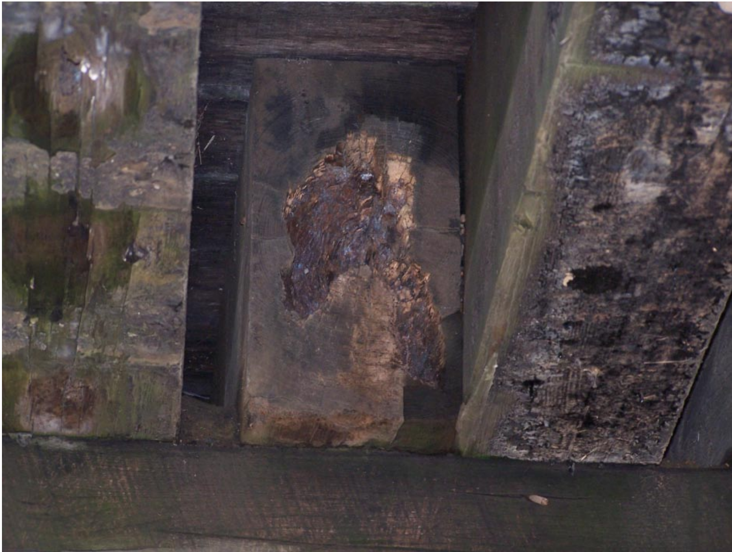
042-C252 DECAYED BEAM END OVER BENT 3 10/20/2011
