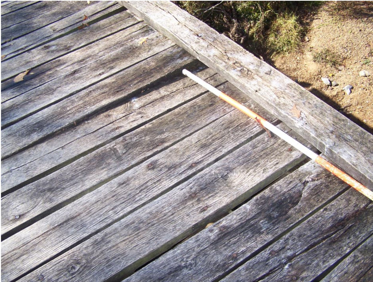
042-C252 LOOSE BOARDS 10/20/2011
